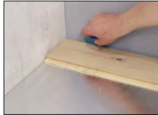
Centre/angle the installation area and adjust the first row of planks by cutting it to size.
